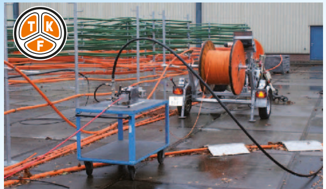
Picture 2: Test circuit for blown cable installation at TKF site
