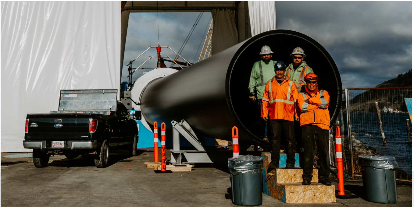
Cover Image: Concrete ballasts were used to anchor the butt-fused HDPE pipe to the ocean floor. Above: Employees in British Columbia stand inside the largest HDPE pressure pipe to be used in North America.
