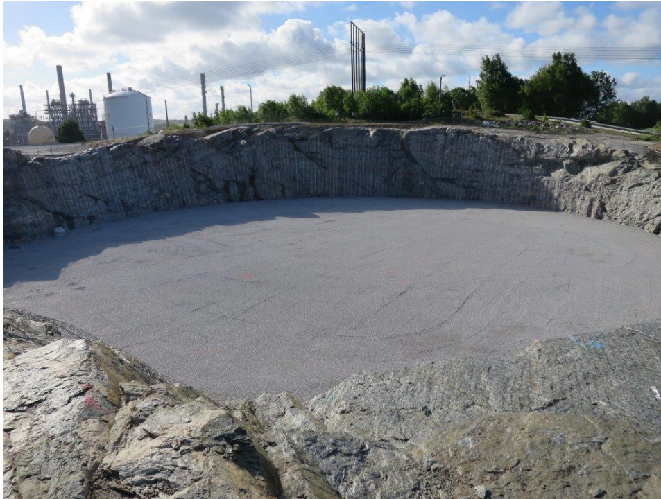
Ground preparations for a new purpose-built, fully refrigerated ethane tank at Borealis site in Stenungsund have started. © Borealis
