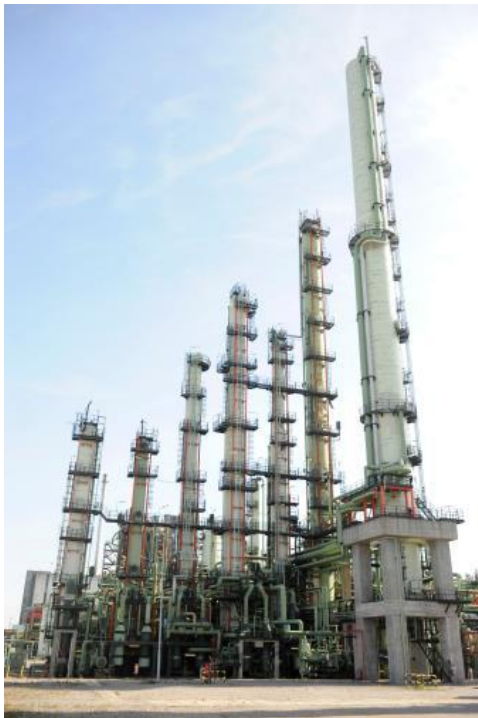
Photo: Borealis cracker in Porvoo, Finland. ©Borealis
