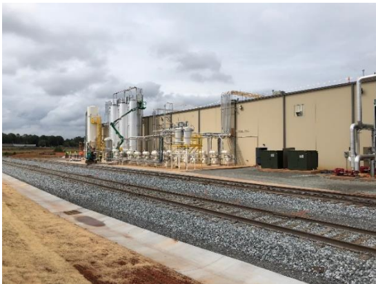
Photo: Borealis' new polypropylene compounding plant in Taylorsville, North Carolina, US. Photo: © Borealis
