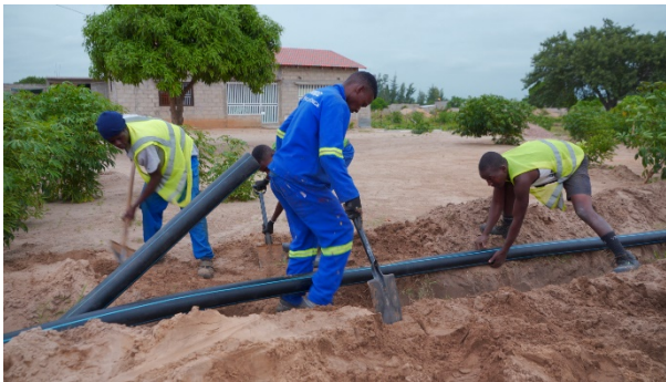
Photo: The works carried out included constructing water supply networks using HDPE PE100 pipes, repairing existing water tanks, training the SSOs’ staff to manage, operate and maintain pipeline systems, and supporting FIPAG so it could more effectively monitor the water quality the SSOs deliver.
